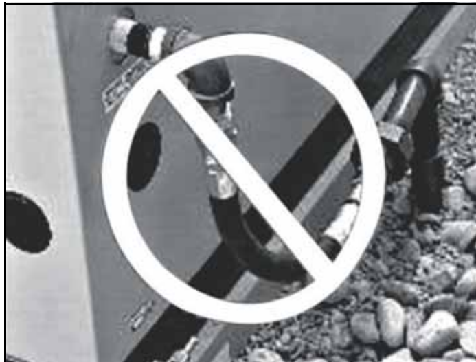
Figure 5-4. Incorrect Routing of Flexible Hose
