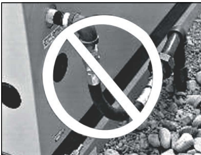
Figure 5-4. Incorrect Routing of Flexible Hose
